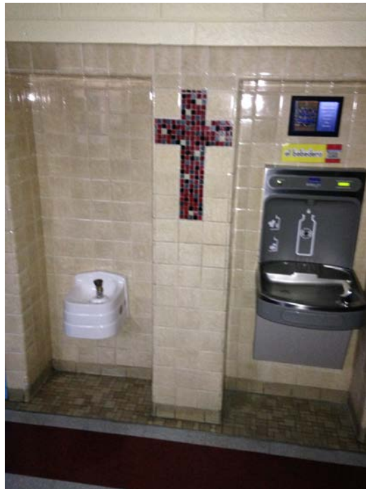
WATER BUBBLER IN SUBJECT BUILDING (SV-WB-02)
