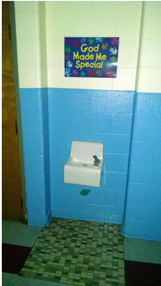
WATER BUBBLER IN SUBJECT BUILDING (SV-WB-03)
